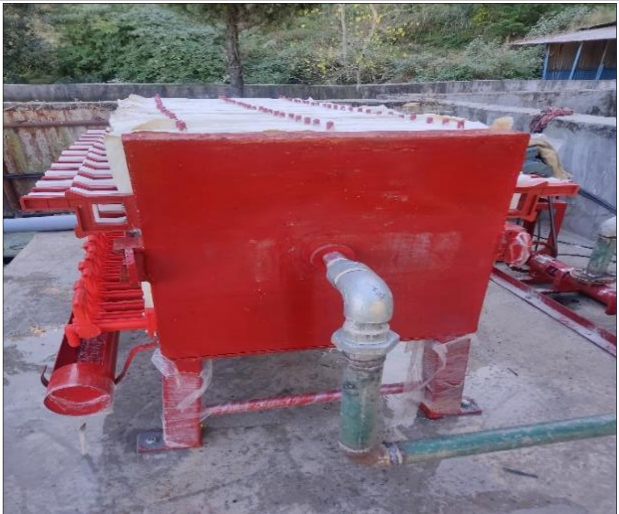
Installed new Hydraulic filter press at township STP, to reduction of evaporation and fast drying process of sludge in rainy seasons
